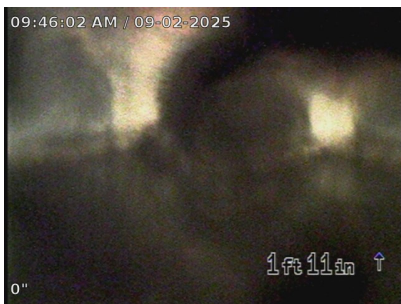
Camera removed from drainfield B. Showing distribution box.
