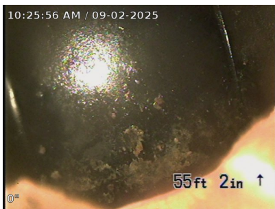
End of front line inside septic tank. The front line was found to be clear of obstructions and breaks.
