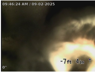
Camera removed from PVC back line.
