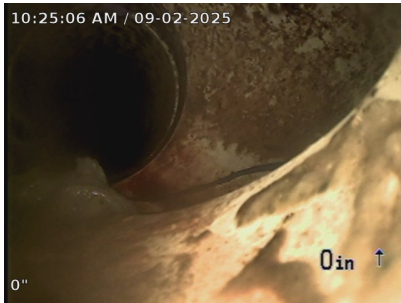
Entry point PVC cleanout in basement wall at back of house. Beginning of cleanout.
