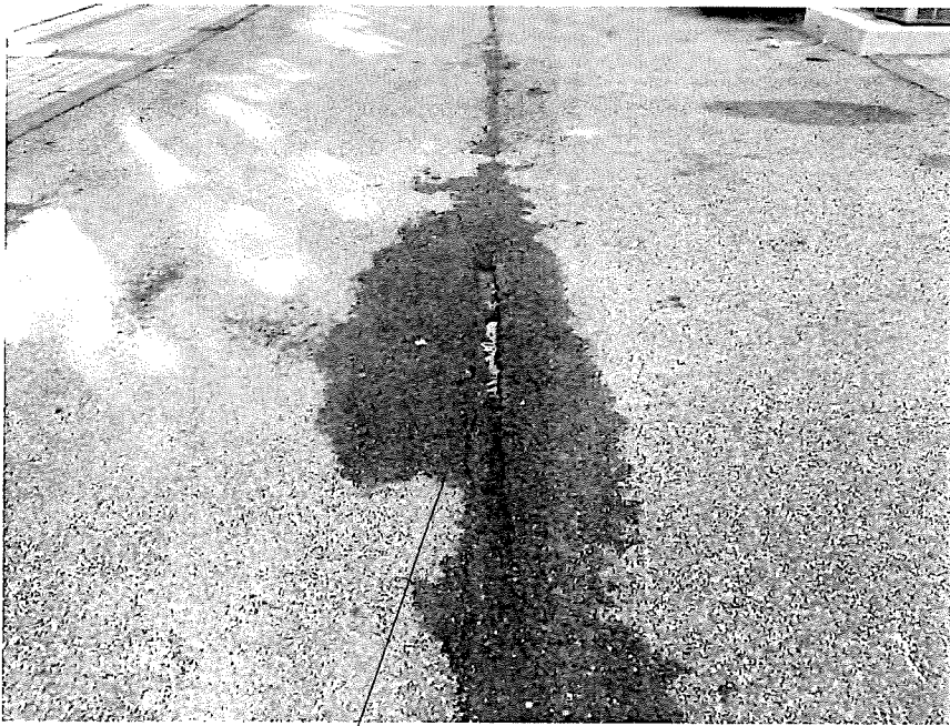
Photograph 18 – Deteriorated pavement along simple crack in asphalt pavement
