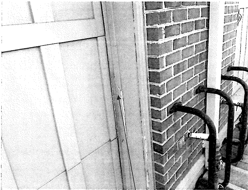
Photograph 14 – Broken trim at garage at 2323-5 Boston Street
