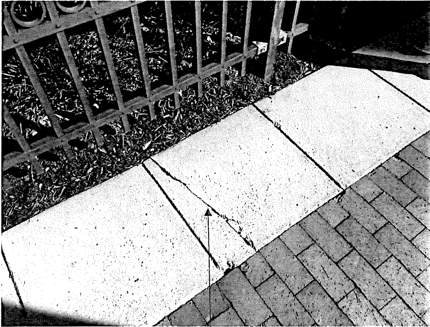
Photograph 30 – Crack in promenade concrete boarder
