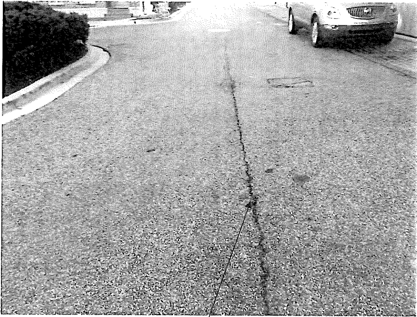
Photograph 17 – Simple crack in asphalt pavement
