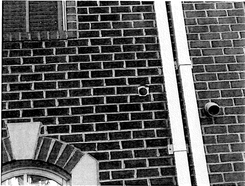
Photograph 5 – Missing dryer vent at 2319-3 Boston Street
