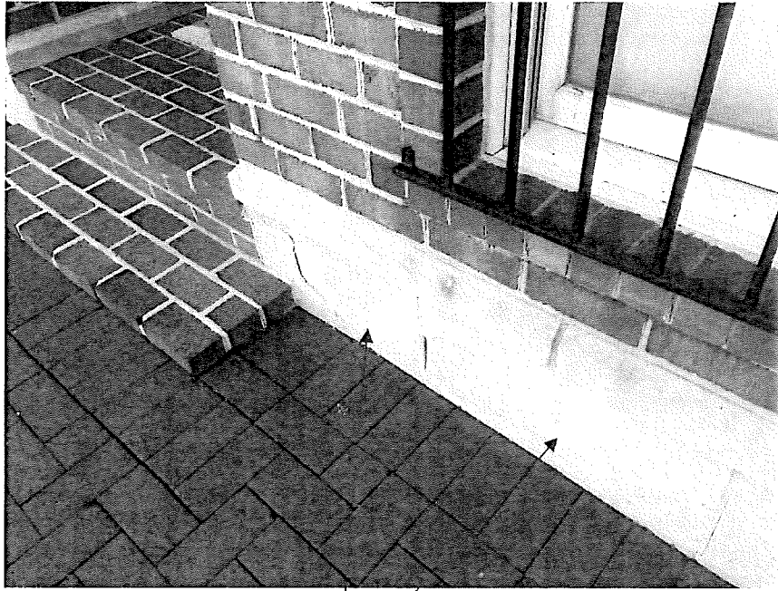
Photograph 9 – Deteriorated precast stone masonry units at ground level
