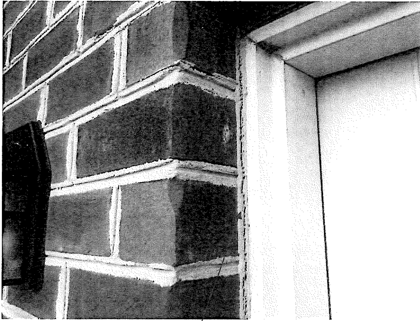
Photograph 13 – Deteriorated sealant at perimeter of door
