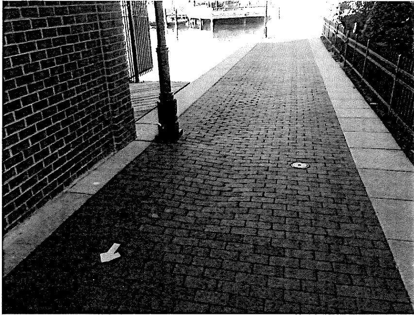
Photograph 29 – Sunken area of brick pavers in promenade at the north corner of the property
