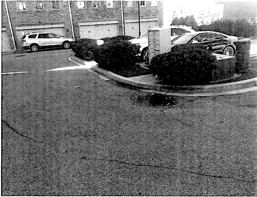
Photograph 21 – Area of ponded water in asphalt pavement
